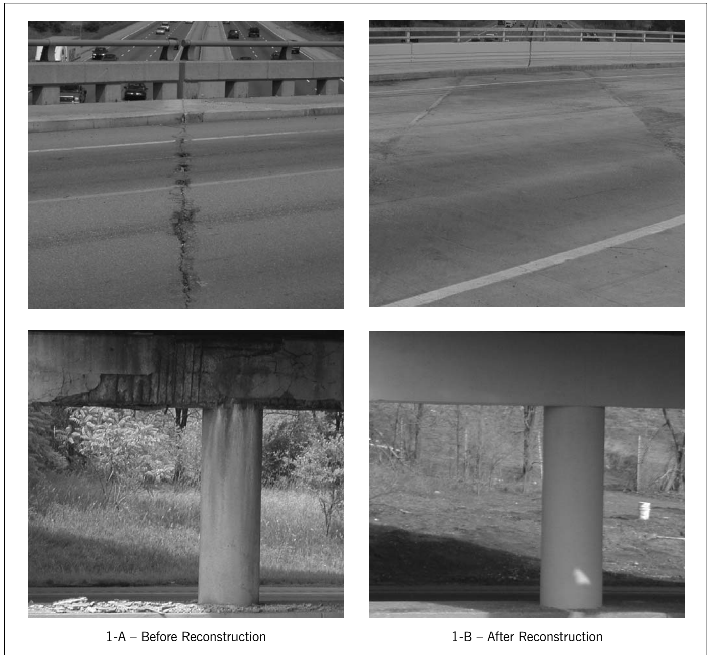
Figure 1. Slab and Support on Grove Street Bridge in Ypsilanti, Michigan, Before and After Reconstruction.
